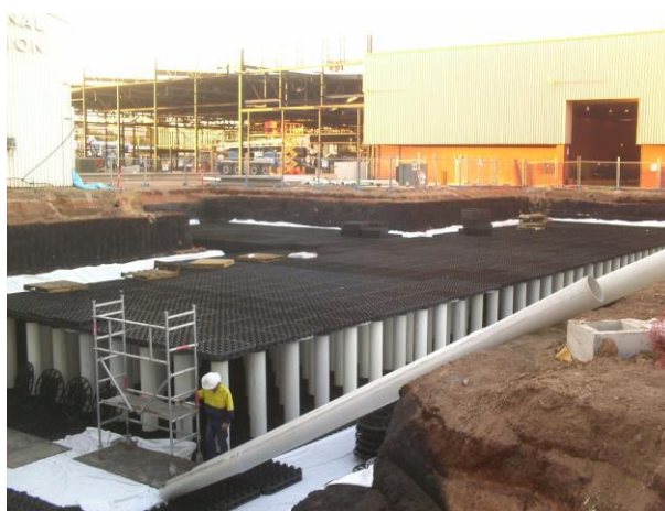
Figure 5 – Invisible Structures Rainstore 3 Tank
