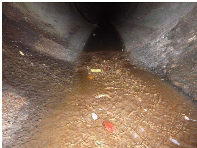
Figure 9: Baseflow observed in 1650mm drainage line
