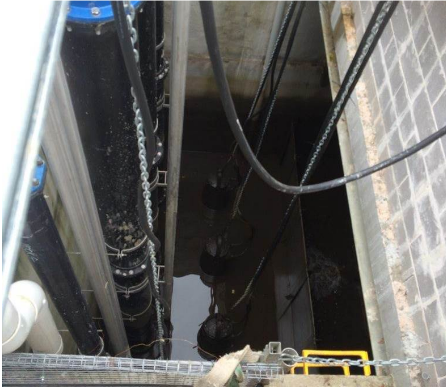
Figure 9: Pumpwell with three large pumps
