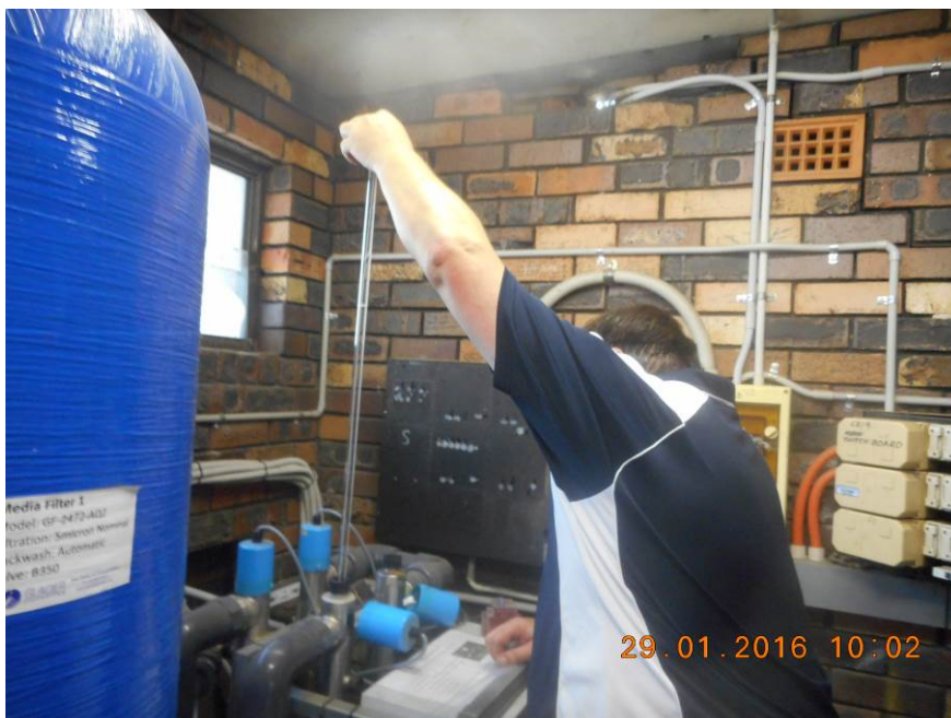
Figure 3: Operation and maintenance of UV lamps
