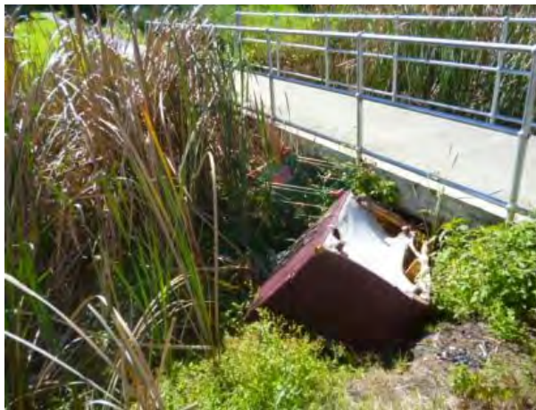
Figure 1 - Upstream pedestrian bridge with sedimentation, vegetation and illegal dumping.
