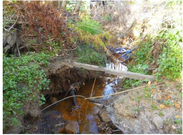
Figure 8 – Evidence of scour and debris within channel
