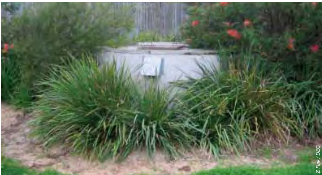
Irrigation storage tank, Powells Creek Park
