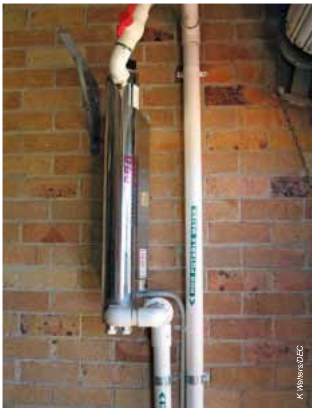
UV disinfection unit at Greenway Park stormwater reuse scheme, Cherrybrook
