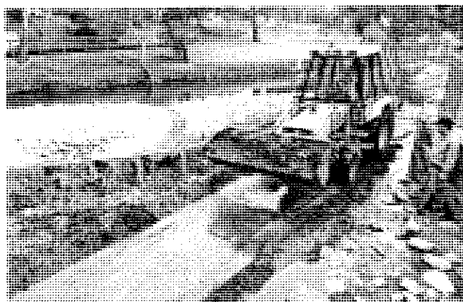
Figure 8.12 Excavators can be used to clean above-ground GPTs. Adelaide, South Australia (source: A. Thomas)
